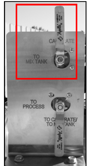
Pumping liquid into the top of the calibration tube for calibration purposes.
