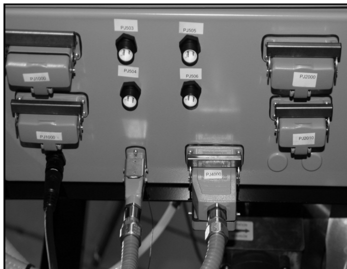
Main Treater Panel Cord Connections
