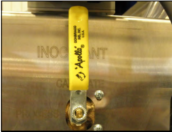
Pump #2 Pumping Liquid to Calibration Valve
