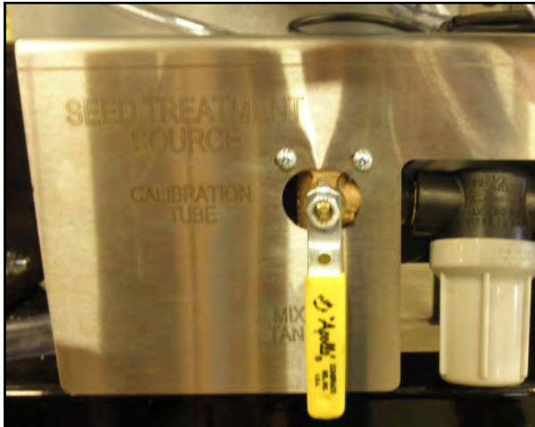
Pump #1 Drawing from bottom of Mix Tank
