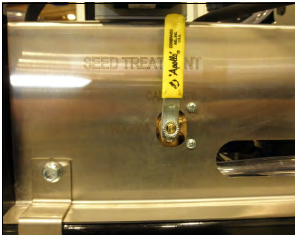
Pump #1 pumping liquid to valve on top of mix tank.
