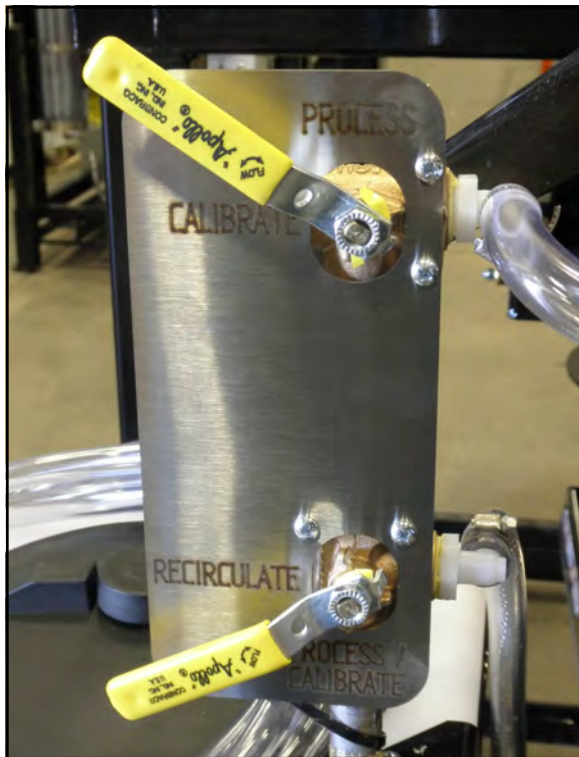
Left Tank Source Valve
