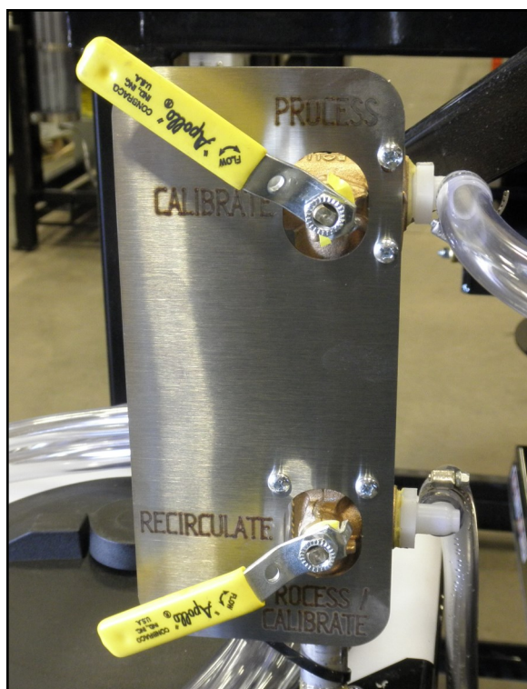
Left Tank Source Valve
