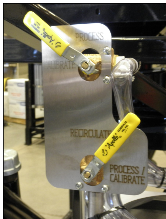
Right Tank Source Valve
