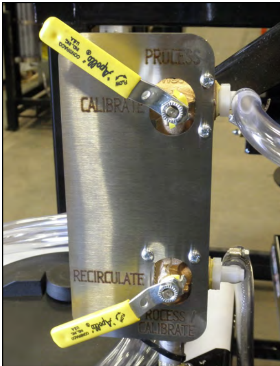
Left Tank Source Valve
