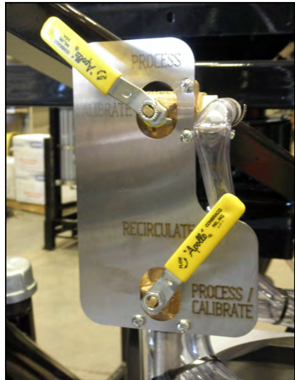
Right Tank Source Valve
