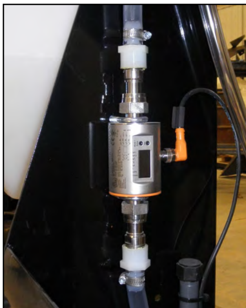
Volumetric Flow Meter
