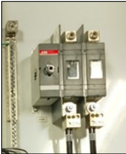
Control Panel Disconnect and Ground Bar
